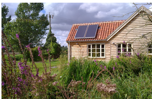
Norfolk Solar, solar thermal installation
