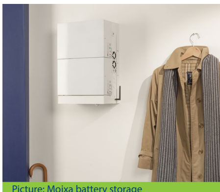
Picture: Moixa battery storage
